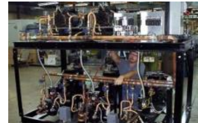
Water Cooled Racks
